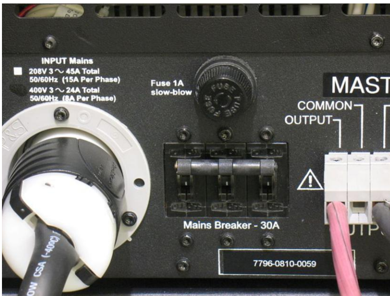
Figure 6.1 Back-Panel Circuit Breakers and Fuse F1 Location
